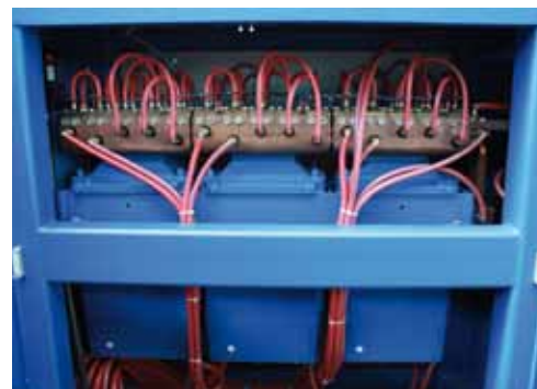
position of transformator and rectifier set
